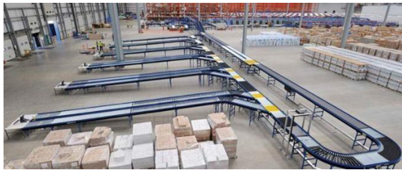
Figure 2: Conveyor and sortation systems
